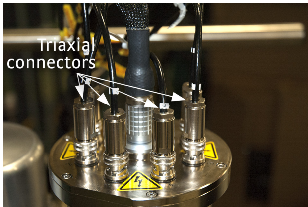
FIGURE 4-36 Attach the primary triaxial cables to the CCR insert
